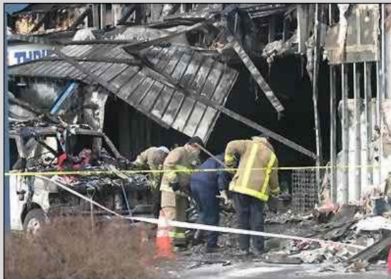
Investigators inspect the damage after fire gutted the Salvation Army Thrift Store on Innes Road.
